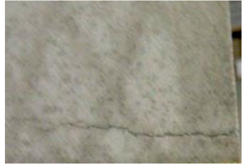
Figure D-10: Fissure
