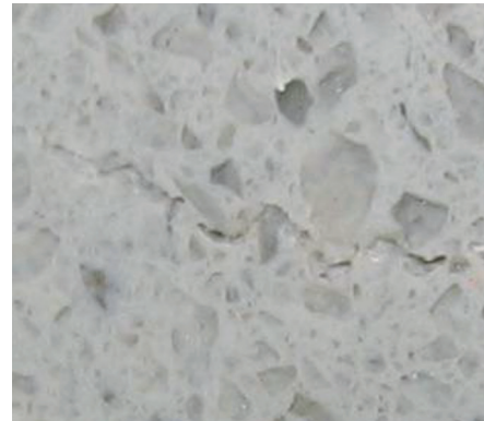
Figure D-11: Surface crack
